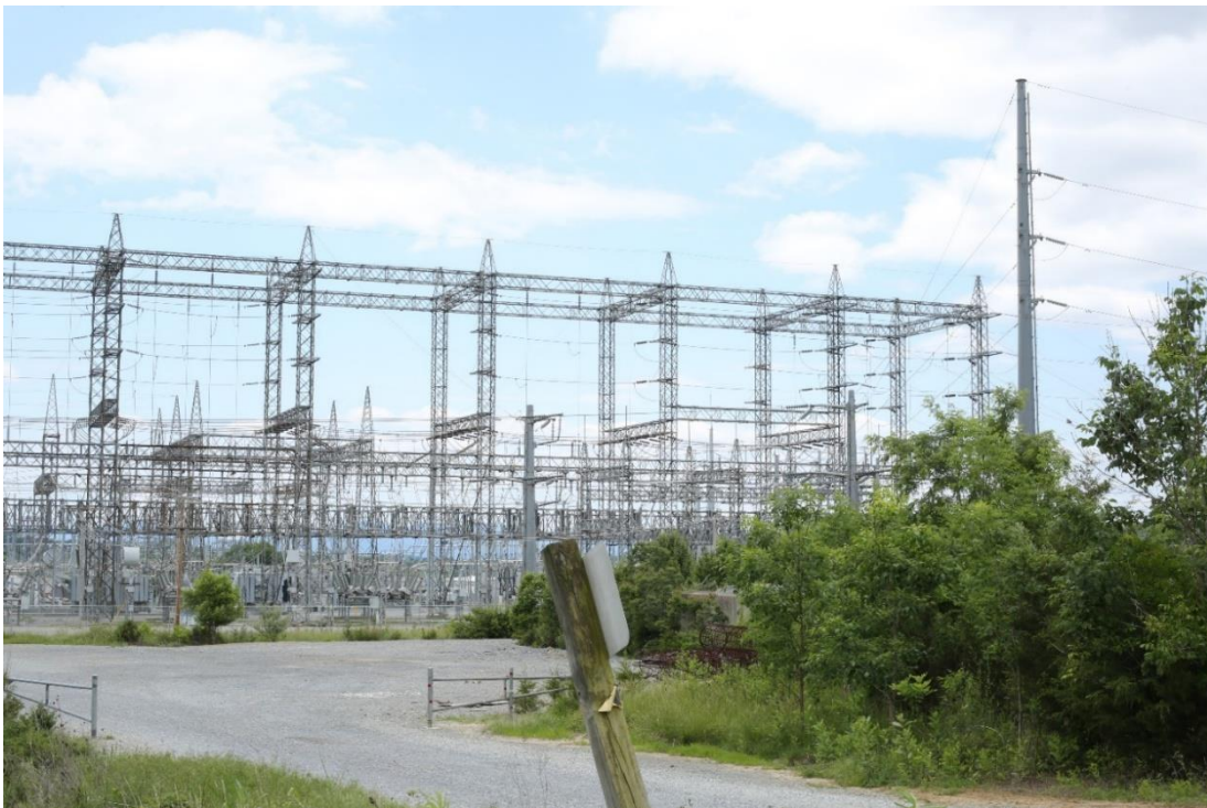
Photo 15: From Norfolk and Western Railway Section (011-5481) toward Cloverdale Substation and the connecting Cloverdale – Windy Pass 138-kV Transmission Line, facing southwest
